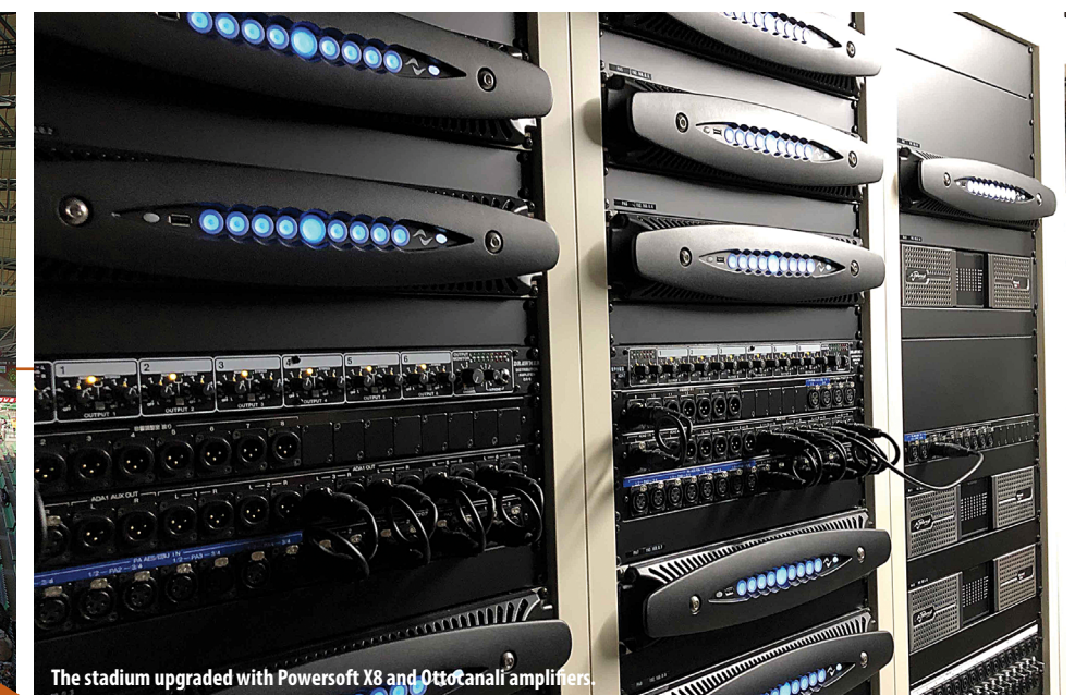
The stadium upgraded with Powersoft X8 and Ottocanali amplifiers.
